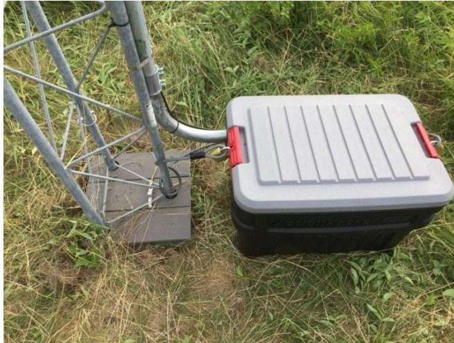
Box containing receiver and batteries
